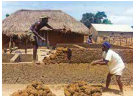
Figura 4.35: Tecnica del Cob (fonte: DEJEANT F., GARNIER P., JOFFROY T., Local materials, materials of the future: Local resources for sustainable cities and territories in Africa , CRAterre, 2021, p. 23).
