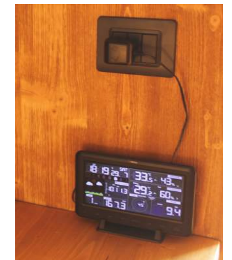
Figure 05.6.17: ICOMAC27 - Micro-climatic station control panel installed on site during the site survey. Source: Picture taken by the author of the thesis
