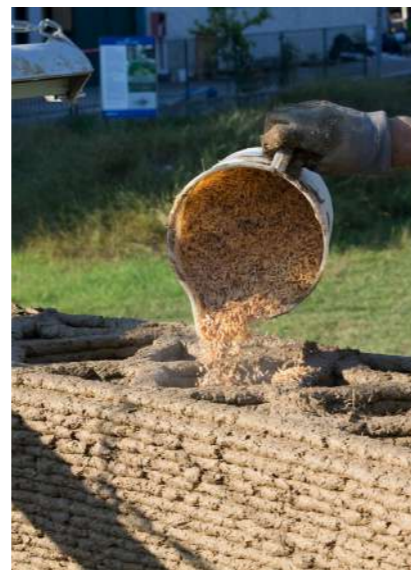
Figure Hk019-20: Wall 3D printing construction process and rice husk infill - by Rice House Source: https://www.ricehouse.it/
