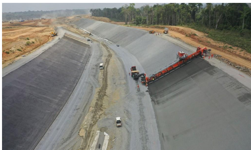
Figure 12b: Hedrace channel under construction: Headrace channel: laying the bituminous lining – April 2022
