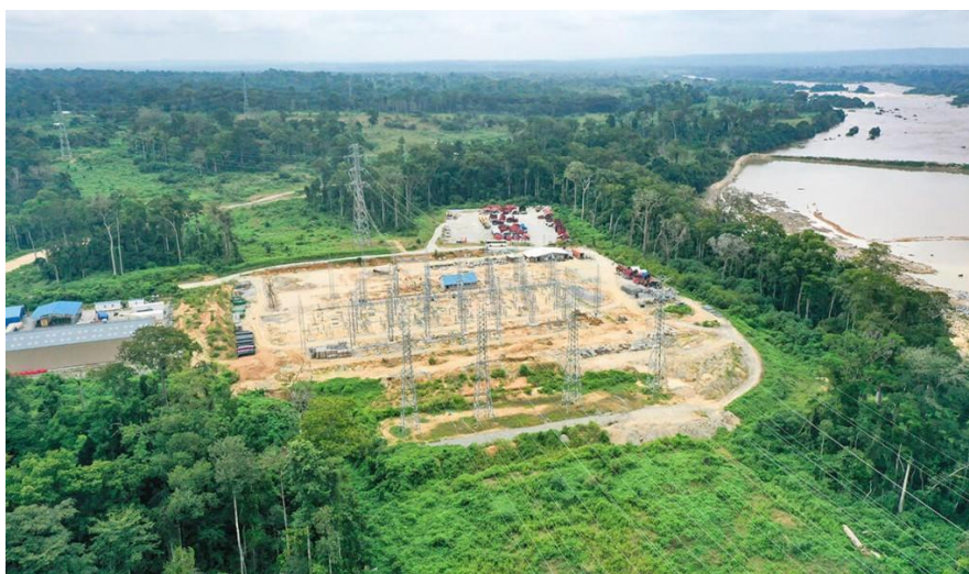
Figure 12d: 225kv transmission line completed: Evacuation station (foreground) – Evacuation lines to Nyom 2 station (background) April 2022
