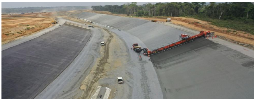
Figure 12b: Hedrace channel under construction: Hedrace channel: laying the bituminous lining – April 2022
