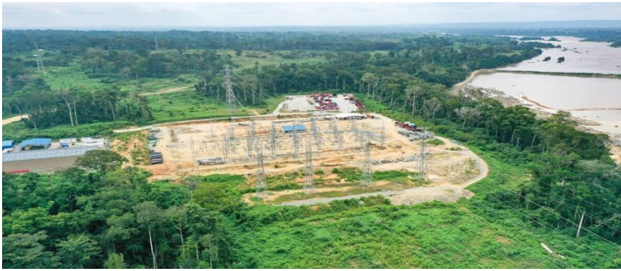
Figure 12d: 225kv transmission line completed: Evacuation station (foreground) – Evacuation lines to Nyom 2 station (background) April 2022
